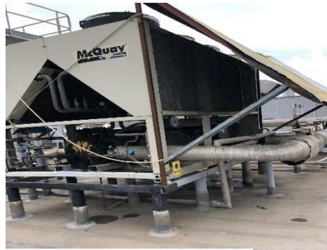
Figure 7. Technical area with a risk of head collision on the roof Source: Author's own work.
