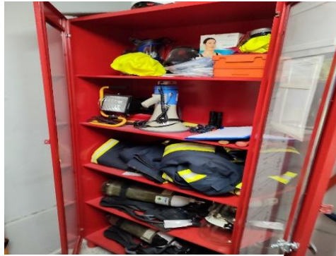
Figure 4. An inspected fire fighting equipment (sample application) Source: Author's own work.
