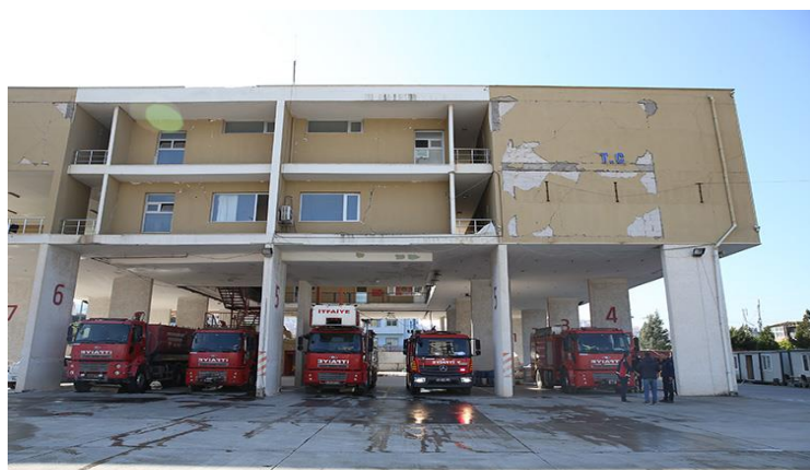
Picture 1: Iskenderun Fire Brigade Building damaged during the earthquake
